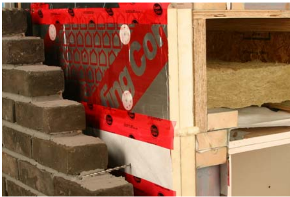
Continuous exterior insulation minimises thermal bridging and leaves the stud cavity empty, making it easier to install services
